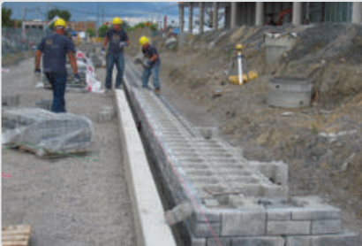
Continue the installation of stabilizing blocks. A level base course and well-aligned blocks allow rapid installation of subsequent rows with no significant repositioning of elements already in place
