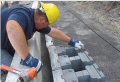
Place the first stabilizers and facings, perfectly aligned using a mason's line
