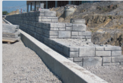
End rows with cascading finished returns to confer excellent stability to the backfill
